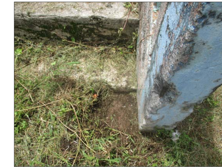
Buried Stair Tread @ bottom of stair
